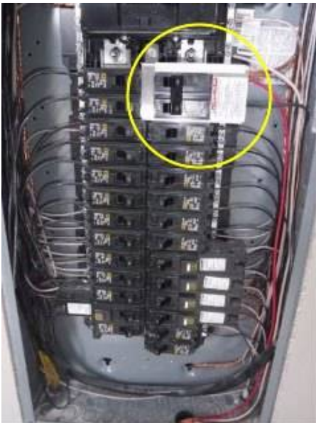
Photo 16-1 Transfer switch for generator connection.
