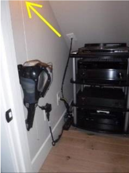
Photo 15-1 Exposed incandescent light bulb fixture in the audio/video cabinet.
