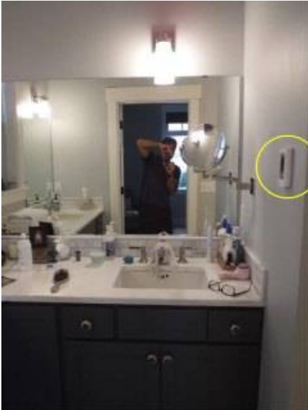
Photo 21-1 Floor heater control head in master bath.
