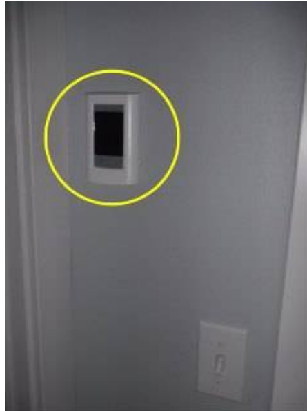
Photo 21-2 Floor heater control head in second floor bath.
