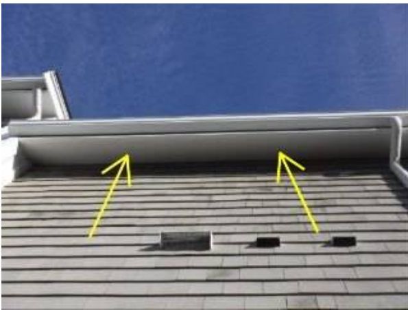
Photo 12-1 A view of one portion of the structure representative of the entire structure. No soffit vents installed.
