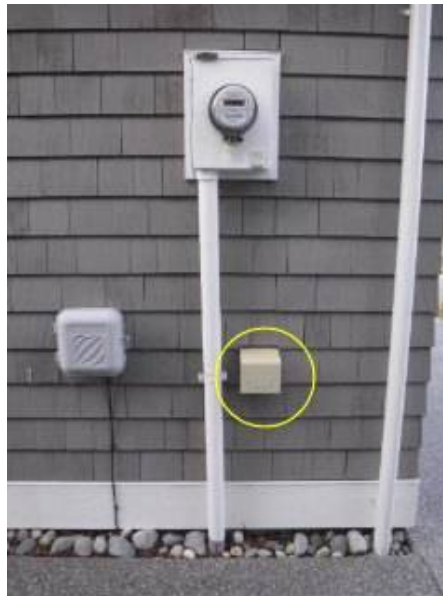
Photo 16-2 Outside generator receptacle at southeast corner of garage.
