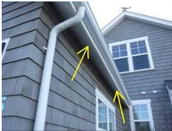
Photo 12-2 Another view of a soffit showing no vents.
