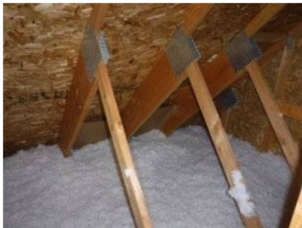
Photo 13-2 Lack of secure footing in the attic limited the inspection to viewing from the access space.
