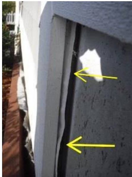
Photo 8-2 View of gap between siding and foundation exposing wooden substructure at the southwest corner of the building.
