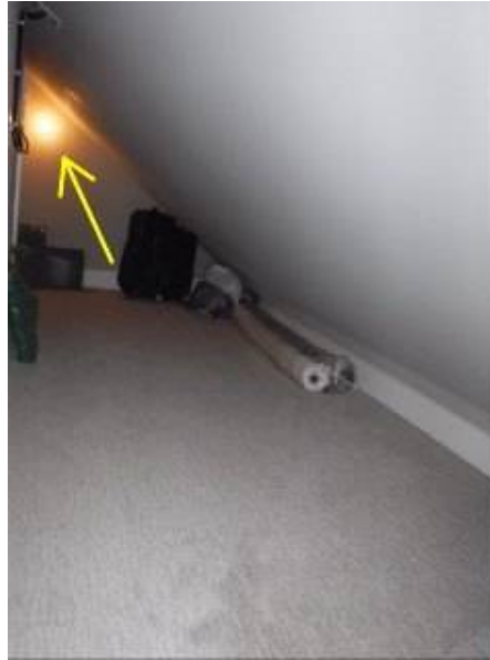
Photo 15-2 One of two exposed incandescent light fixtures in the storage closet in bonus room on second floor.
